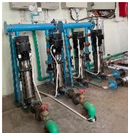
Figure 9. Clean Water Installation System at GKB 2
