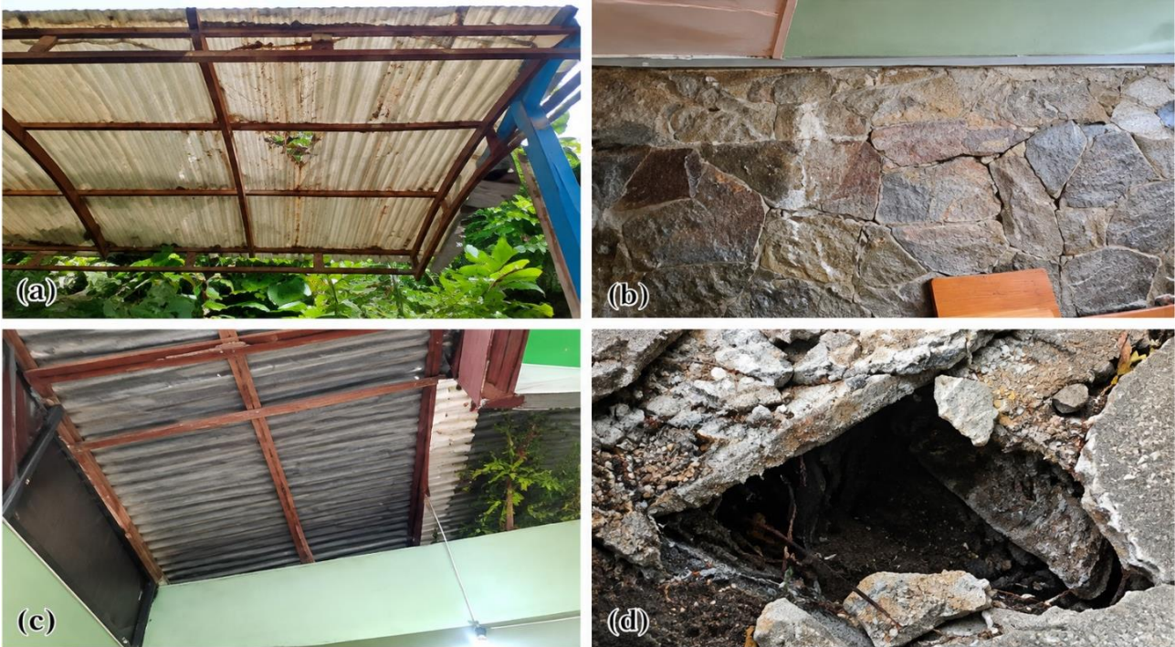
Figure 2. (a) The polycarbonate roof has holes and is leaking; (b) The school fence wall is cracked; (c) The roof over the walkway has holes and leaks; (d) The school access road is full of potholes and severely damaged
