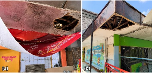
Figure 3. (a) The damaged ceiling at TK ABA25, covered with a banner due to a leaky roof; (b) Inspection and repair of sporadically damaged ceilings
